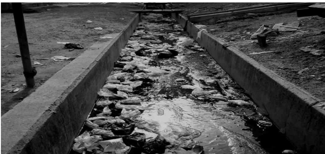
Plate 1: Waste dumped in drainage channel in Sabon gari Source: Field Survey, 2019
