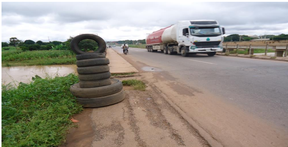
Plate 2: Narrow and dilapidated Bridge at Goningora (Kaduna-Abuja Road)
