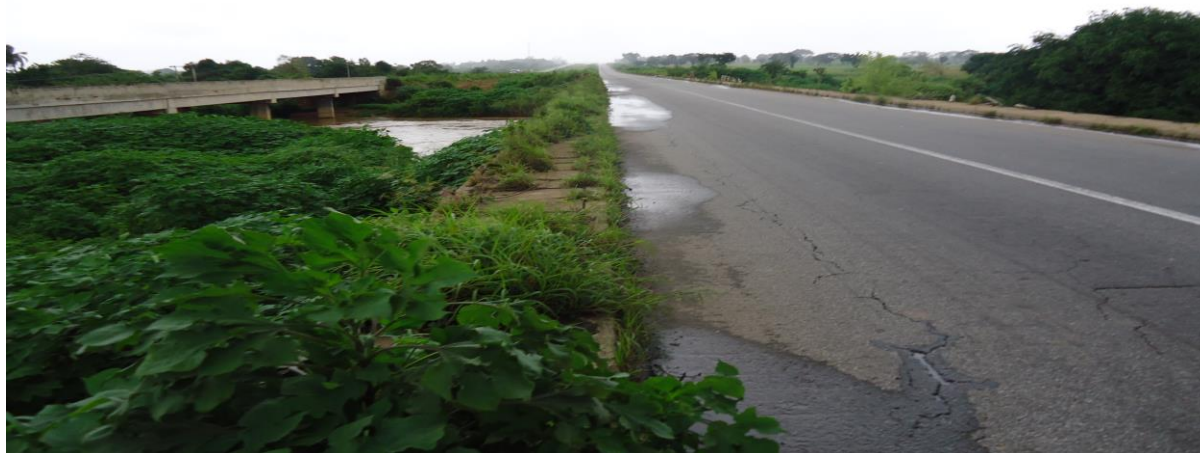
Plate 5: Narrow Bridge and Wash-out at Gidan Busa along Kaduna-Abuja Road
