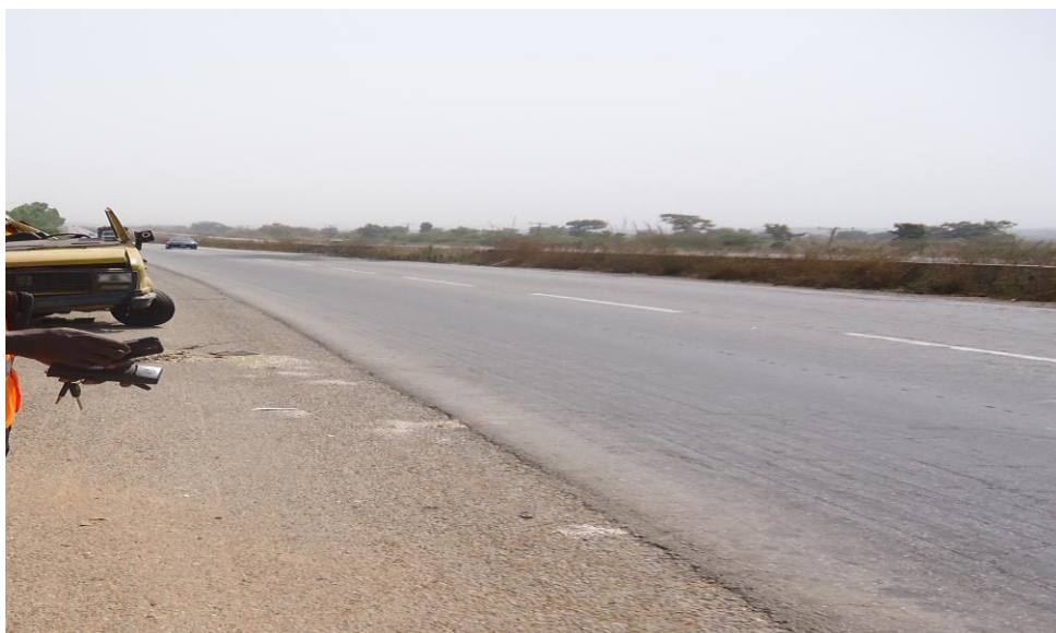
Plate 3: Potholes and sharp bend at Sabon Gayan along Kaduna-Abuja Road
