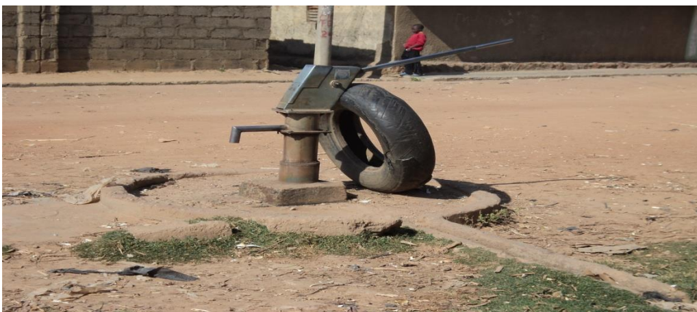
Fig. 3: A non-working borehole on Kwara road, Dogarawa
