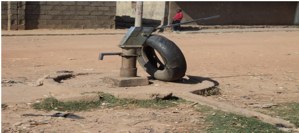
Fig. 2: A non-working borehole on Kwara road, Dogarawa
